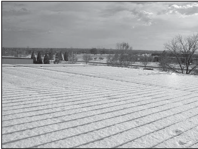
Figure 3 – Submerged SSMR after hailstorm.
